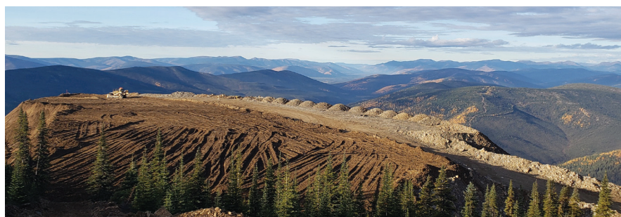
Pilot scale cover trial overview on Platinum Gulch during the construction phase of the Eagle Gold Mine.
