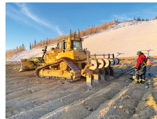
Laying out heap leach emitter tubing on the mine’s heap leach pad.
